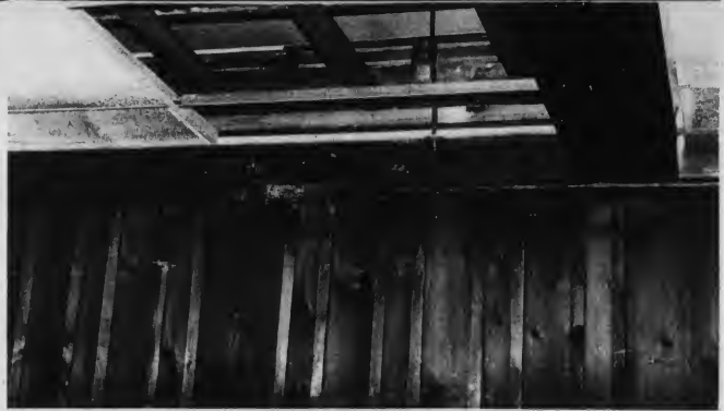
The damaged sprinkler system led to the closing of Beta. Orient/Zuckert
