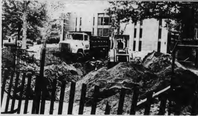
The Kresge Foundation will provide funding for construction of the new library addition. Orient/Pope
