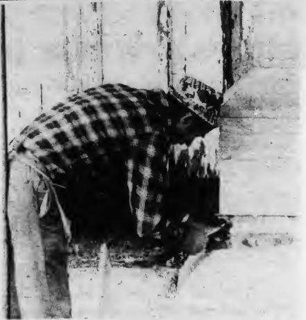
A workman helps out with the nose job. The restoration project will be completed in October.
