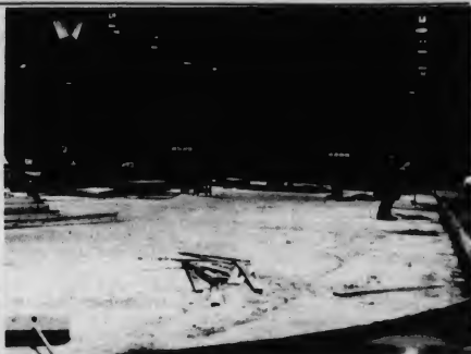
Construction, well underway at the Dayton Arena, should be completed in time for this summer's Clinic.
