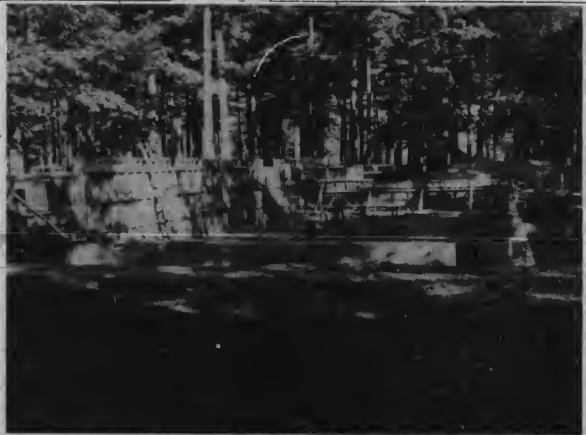
Construction of Coleman Hall began on August 12 and is progressing well as the above photograph shows. The building is being constructed to the south of Hyde Hall near College Street. $450,000 has been given by Mrs. James Coleman Pickard to construct the dormitory and equip it for 78 students.
