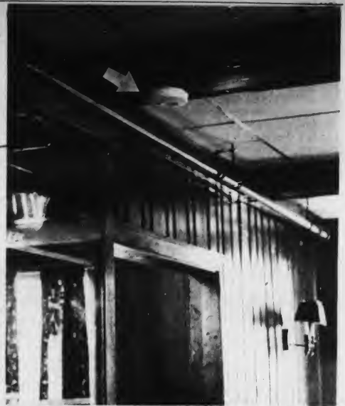
A smoke detector at Beta (see arrow, above) is one of the precautions against fire that the Brunswick Fire Department compelled Bowdoin fraternities to install. Orient/Thorndike.
