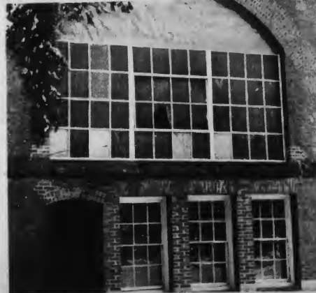
This poor window was a victim of student vandalism.
