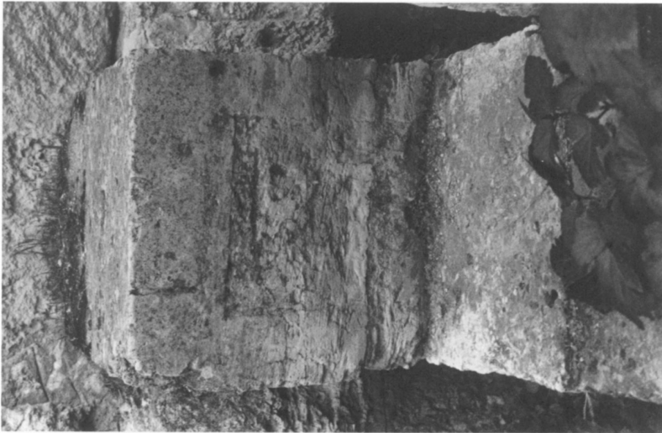
a. Anathyrosis on block of north wall 2 of the Archaic cistern. From west
