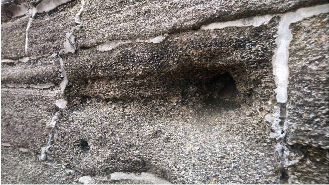
Figure 4: Crumple zones in the coquina walls of the fort Castillo de San Marcos in St. Augustine. Photograph by T. Cavanaugh
