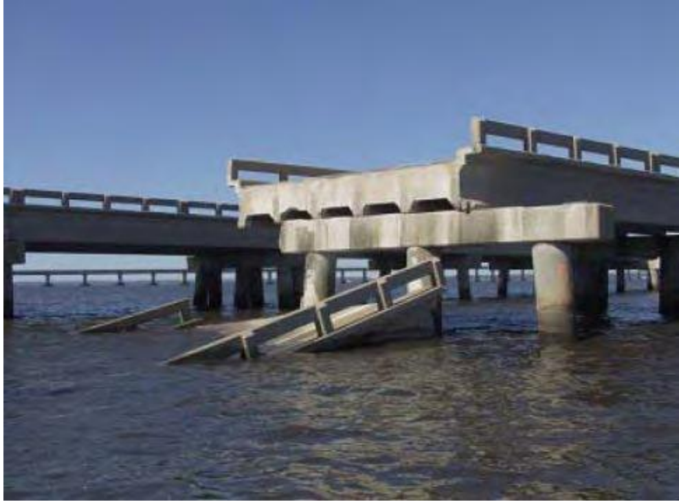
Figure 1-1. I-10 Bridge Escambia Bay spans removed by Hurricane Ivan
