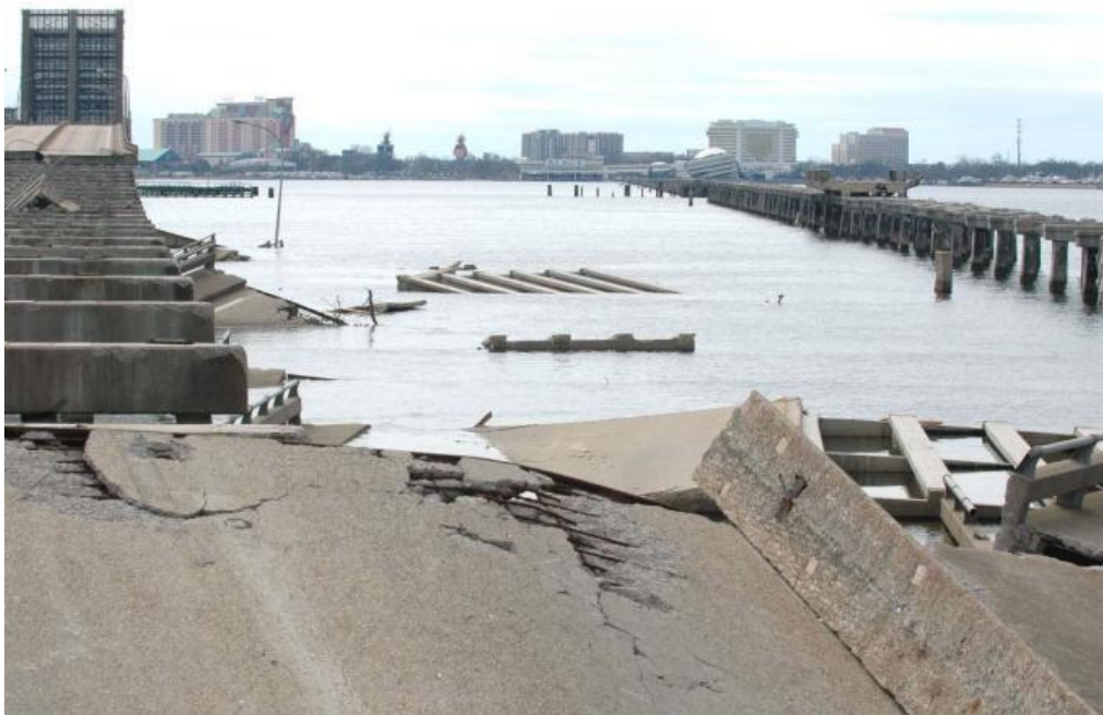
Figure 1-2. Photograph of U.S. 90 Bridge over Biloxi Bay showing bridge deck damaged by Hurricane Katrina
