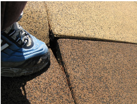
Photo 7: TIL where seams have started to shift.
