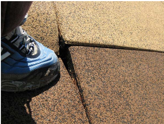
Photo 7: TIL where seams have started to shift.
