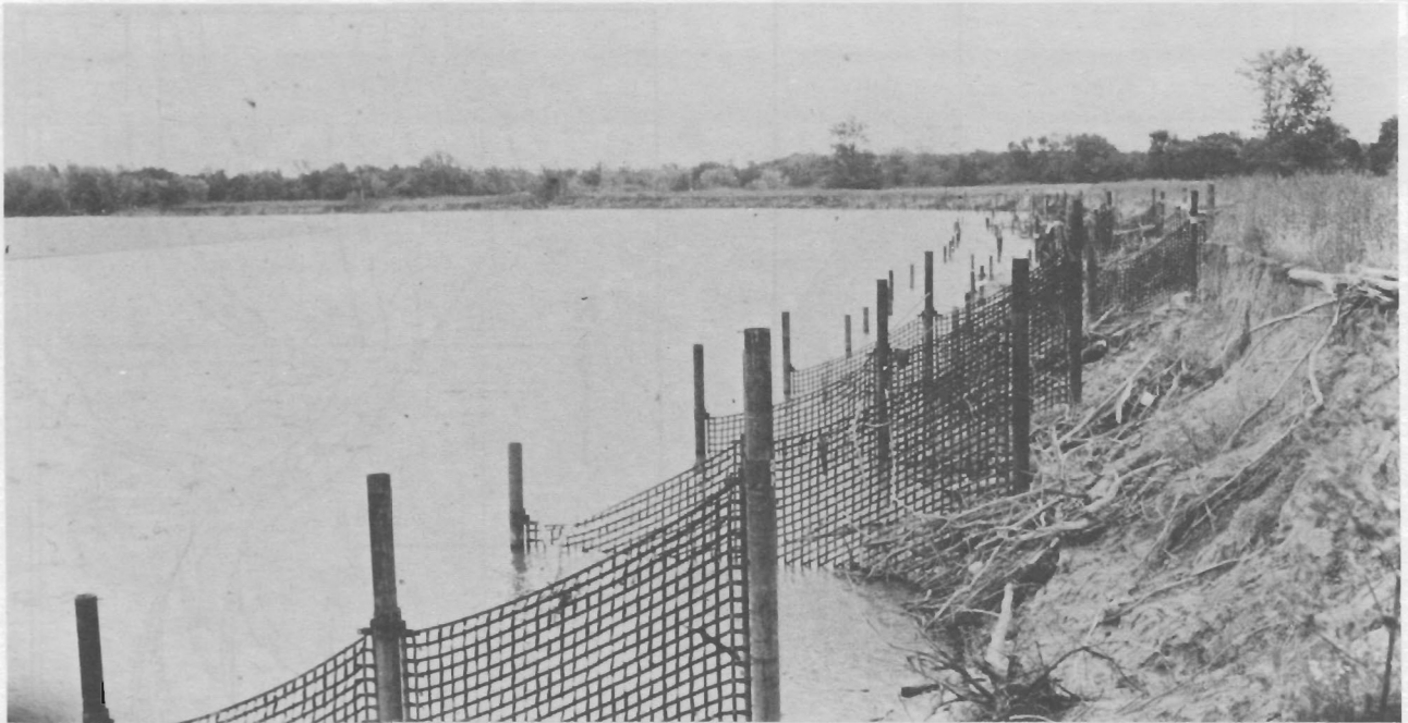
Figure 2. Photograph of part of the east bank of the Wabash River showing permeable jetties installed in 1985-86 by ERCON, Houston, Tex., as preventative of further bank erosion north of New Harmony. Photograph by Shaver (1986).
