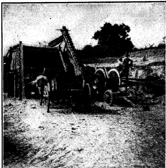
Side view of stone crusher, showing elevator and box dump for loading the crushed stone in the wagons.
