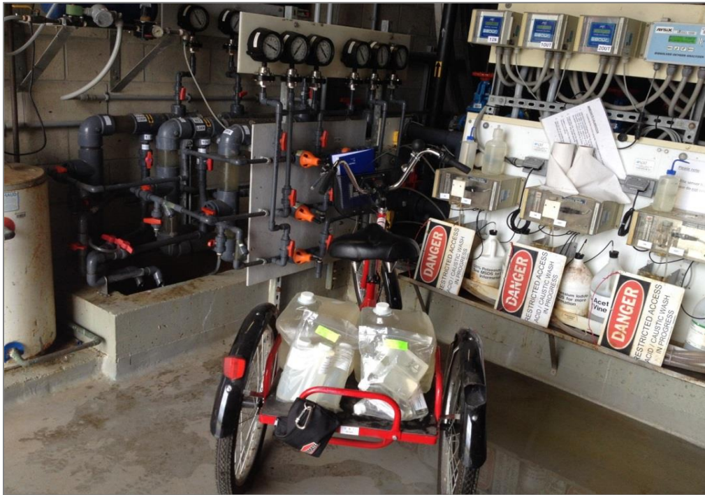
Figure 3. 3: Sampling from the effluent of a WWRF (June 2014)
