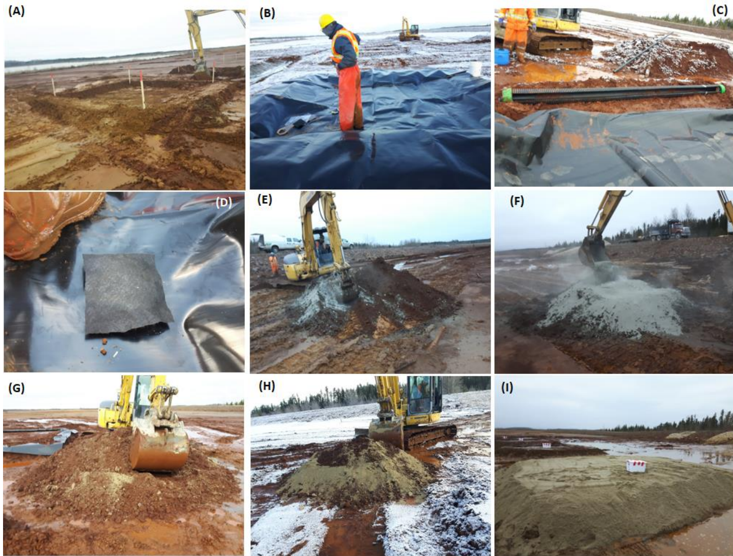
Figure 7.1 : Images showing field cells construction and amendments mixing with oxidized tailings (A, B, C and D : cells excavation, geomembrane and drains installation, E, F, G, H, I: amendments mixing with oxidized tailings)
