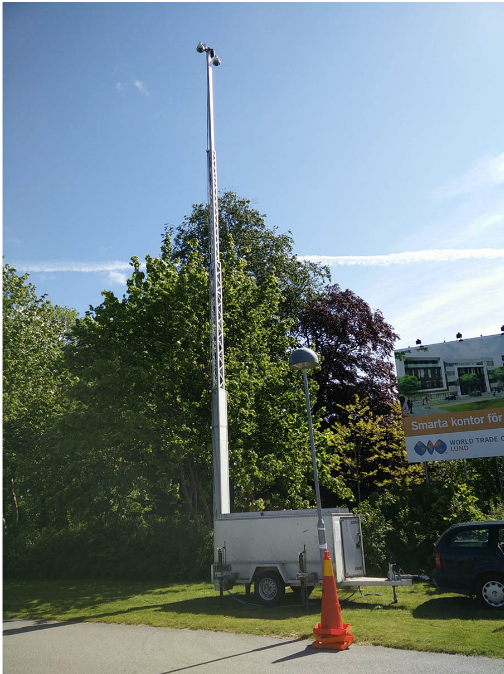
Figure 6.2 Example installation of a trailer-type video data collection unit.
