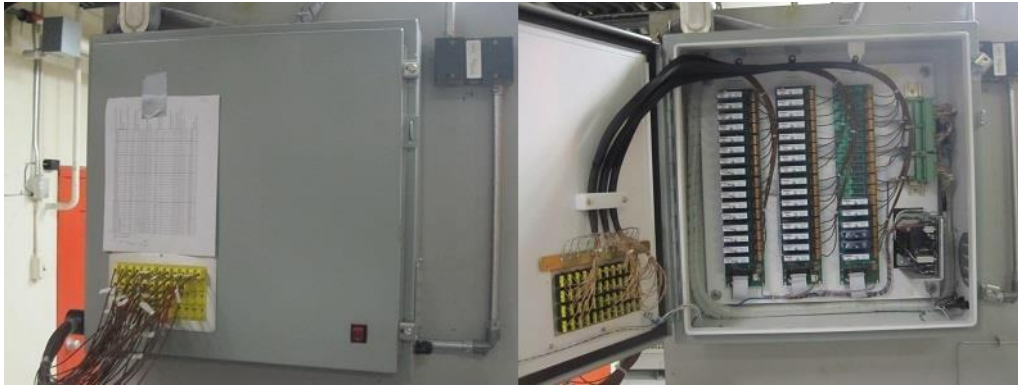
Figure 2.24 Partial view of the temperature measurement panel and the galvanic isolator amplifiers.
