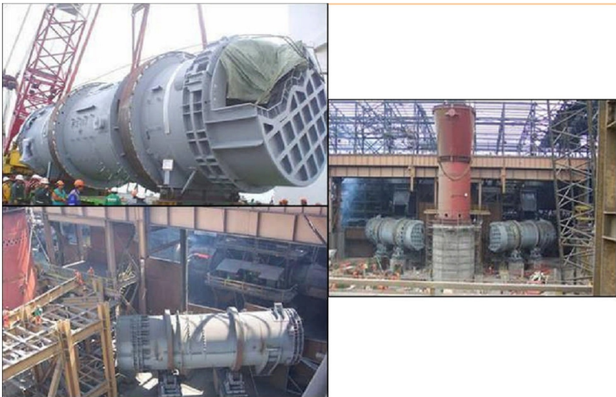
Figure 11.7. Rotary holding furnaces at Ilo copper smelter [398].
