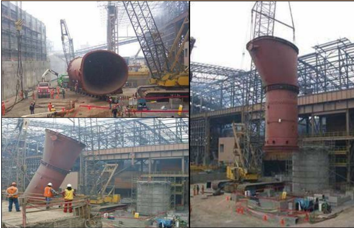
Figure 11.6. The ISASMELT™ furnace installation at Ilo copper smelter [398].
