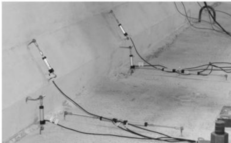
Figure 5-32: Barrier and Slab Crack Opening and Relative Uplift Sensors
