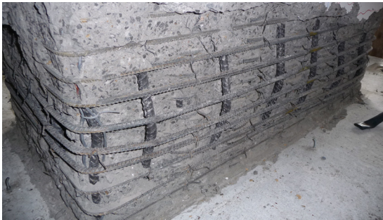
Figure 12. Close-up view of the plastic hinge regions at failure: (a) Spalling of cover concrete and buckling of unsupported longitudinal bars; (b) Specimen S1 after removing of spalled concrete; (c) Specimen S3 after removing of spalled concrete.
