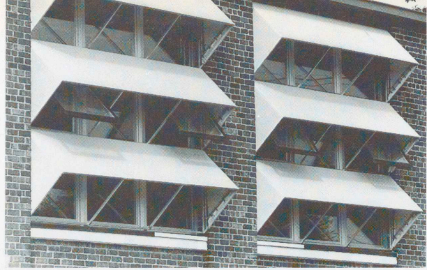
These "awnings" are actually solar screens. Steel tubing and mesh-like cloth were designed specifically to provide a minimum of direct sunlight and a maximum of diffused light.
