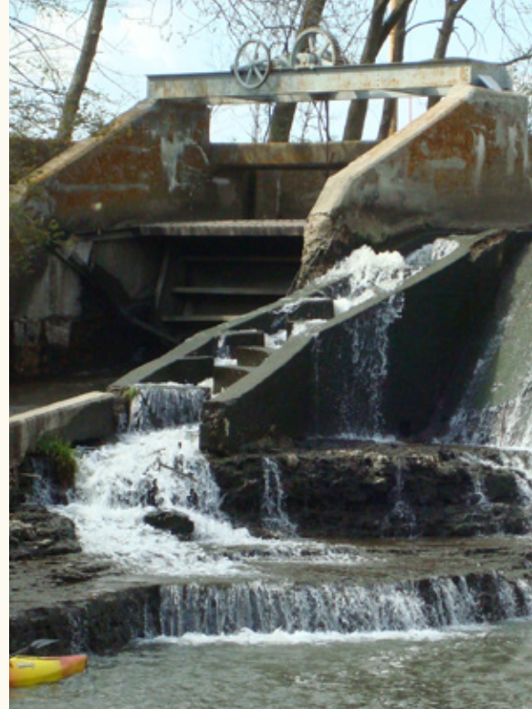
Left and center: images of the interior of the dam, 2002. In center image, note the exposed bedrock near the western end of the dam. Right: close-up image of the Tainter gate and fish ladder, facing northwest (Doug Hawker).
