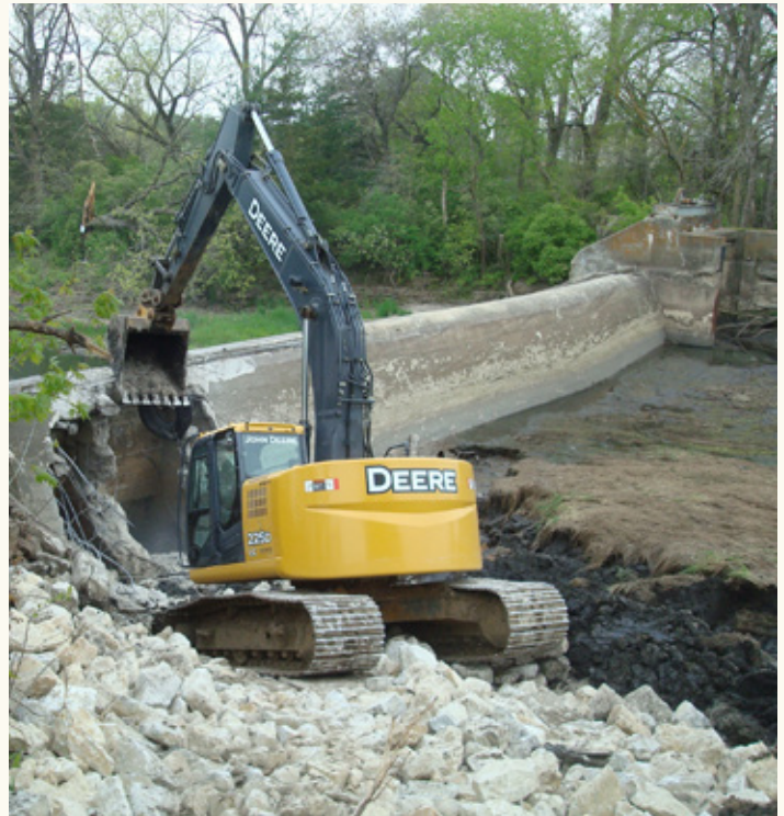
Dam demolition at the eastern end, view to the southwest, May 2017 (Doug Hawker).
