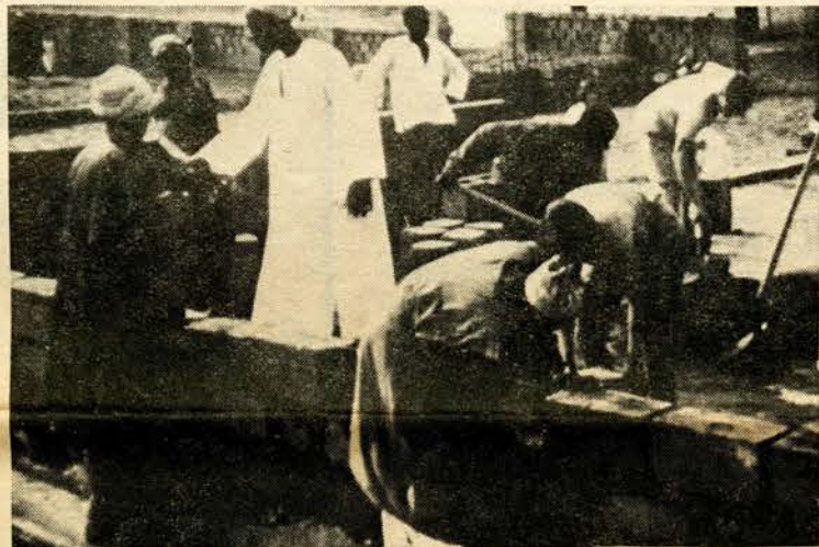
U.S. & Niger students work under supervision of local masons to build a youth center in Tahoua, Niger
