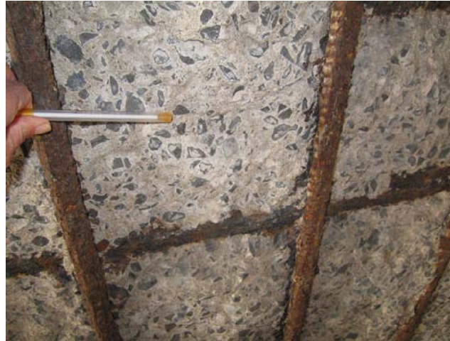
Figure 1. Reinforcing bars exposed by spalled concrete [2]
