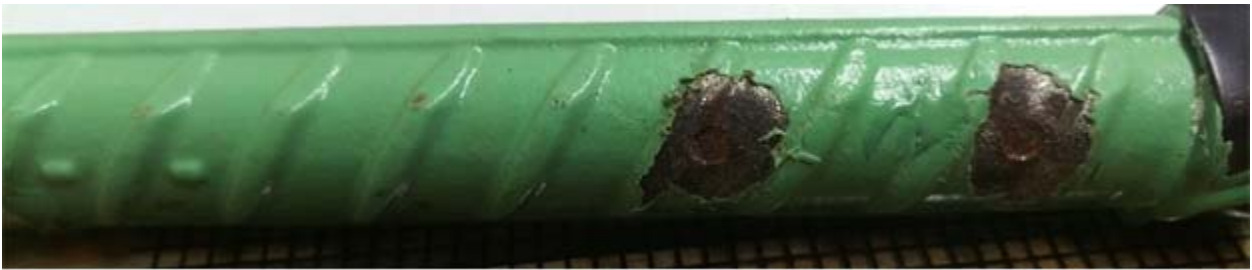
Figure 68 — Rapid macrocell test, anode bar of MMFX-ECR(2%)-5 after disbondment test after 15 weeks
