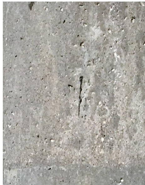
Figure 5.24: Test image for crack width computation
