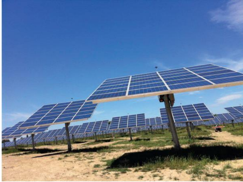
Figure 1.5. Solar cells in a solar farm, South Burlington VT [29]
