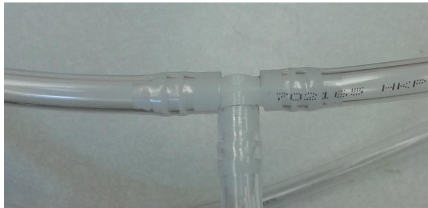
Figure 4 Clear plastic tubing attached to a tee. The top two tubes attach to the static and total pressure ports of the Pitot-static tube while the bottom tube sends this combined reading to the Dwyer manometer.
