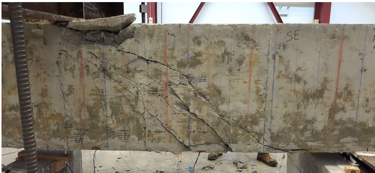
Figure 1.2: Inclined cracks in a reinforced concrete beam
