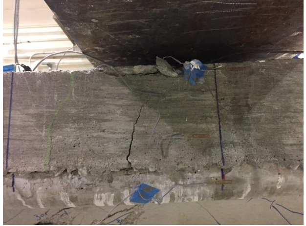
(b) Deck Cracking Below the Loading Point after Failure
