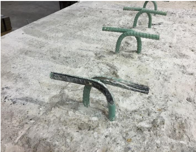
(a) Saw-Cut Damage to Rebar (Girder #3)
