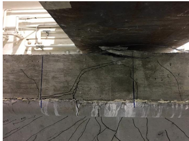
(b) Compression Zone Failure
