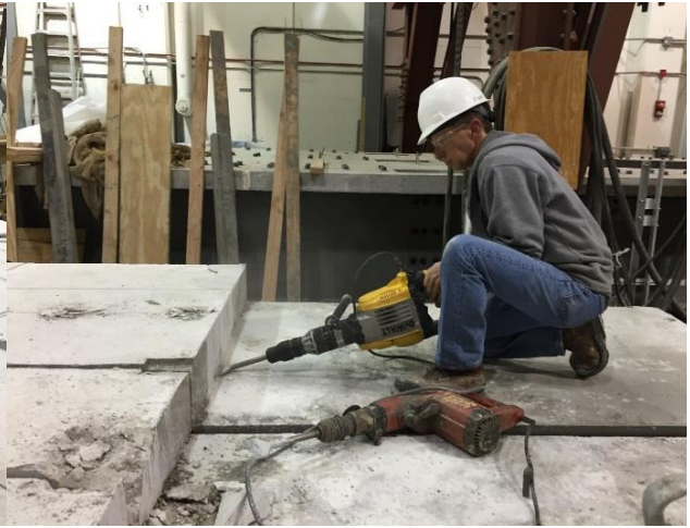
(b) Use of Demolition Hammer at a Low Angle to Break Deck Sections Free
