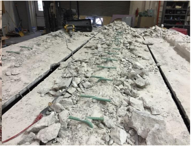
(b) Deck Condition After Use of the 65 lb Jackhammer
