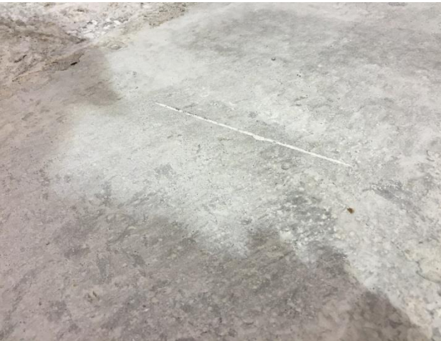
(b) Saw-Cut Damage to the Girder Top Flange (Girder #2)
