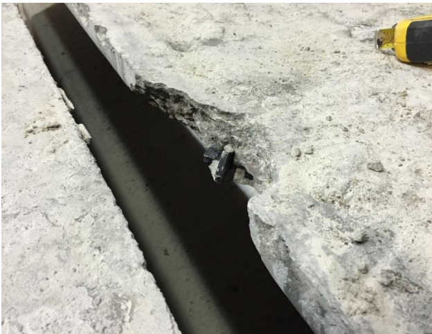
(c) Broken Flange Tip (Girder #3)
