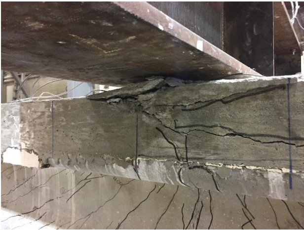
(b) Compression Zone Failure
