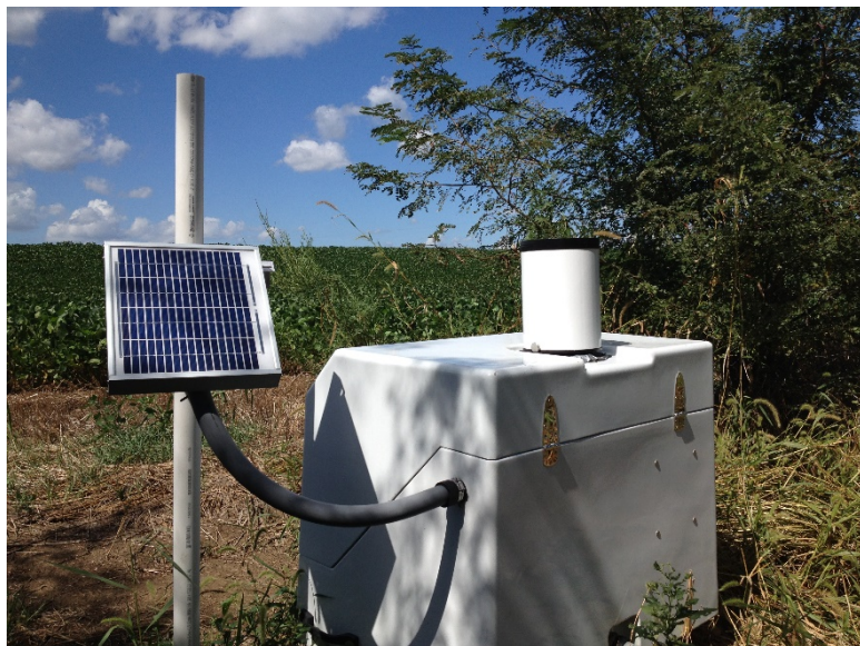
Figure 4. Typical wetland auto-sampling equipment set up 8 .
