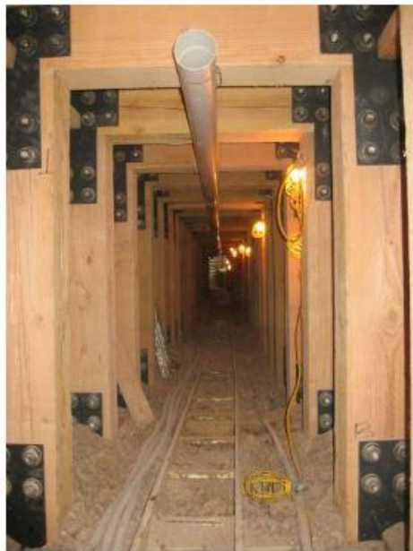
Figure 2: Photograph inside a tunnel that is similar to the tunnel at YPG showing the wood braces, tracks, ventilation pipe and electrical lighting (Image from Sloan et al. (2012))
