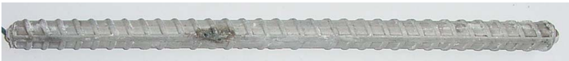
Figure 3.131 – Corrosion products on bars used on top mat of cracked beam specimen CB-2101(2)p-45-1, at week 96.
