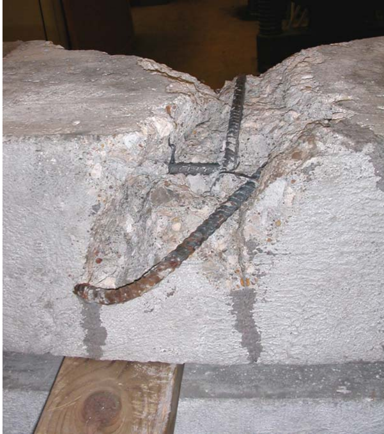
Figure A.27– Top view of Beam 2A after it has been straightened. The dark gray lines are from the epoxy that had been injected into the large cracks prior to straightening.
