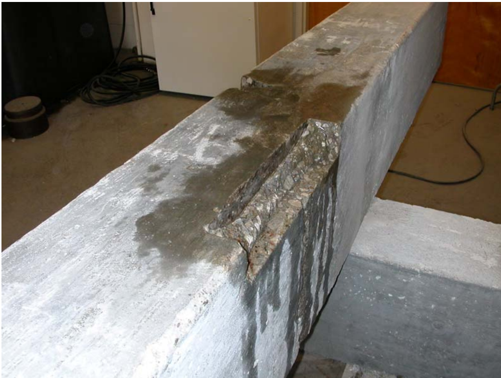
Figure A.31 – The damage on the right side of the top front edge in Figure A- 30 was cut out the same way using a masonry blade on a skill saw.
