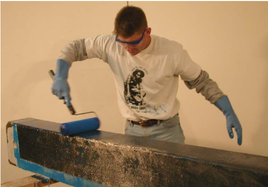
Figure A.48 –The MBrace Saturant was applied on top of the fabric using a medium nap roller. The saturant was applied generously to ensure that the fabric was fully saturated.
