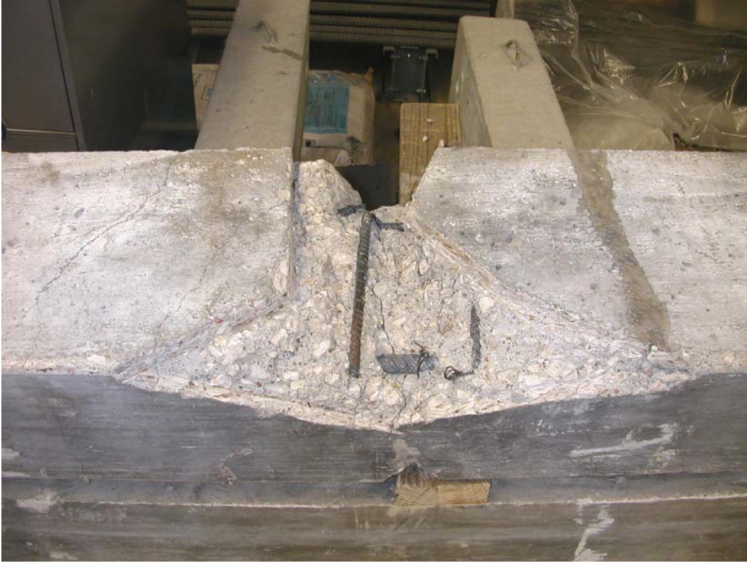
Figure A.28 – The edges around the area in which the high-strength repair mortar was to be placed were cut ½ in. (13 mm) deep using a masonry blade on a skill saw.
