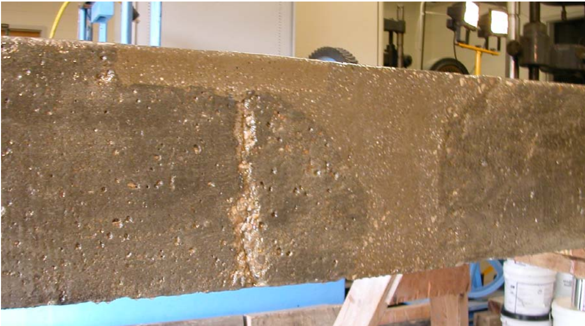
Figure A.40 – The repaired portion of beam 2A could be clearly seen after the primer coat was applied.
