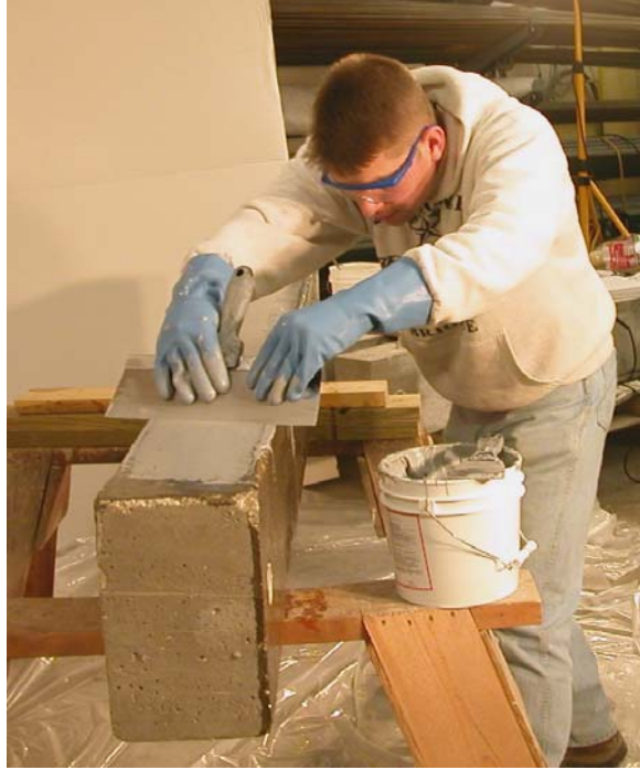
Figure A.43 – The MBrace Putty is applied in a thin coating to smooth the surface of the beam.
