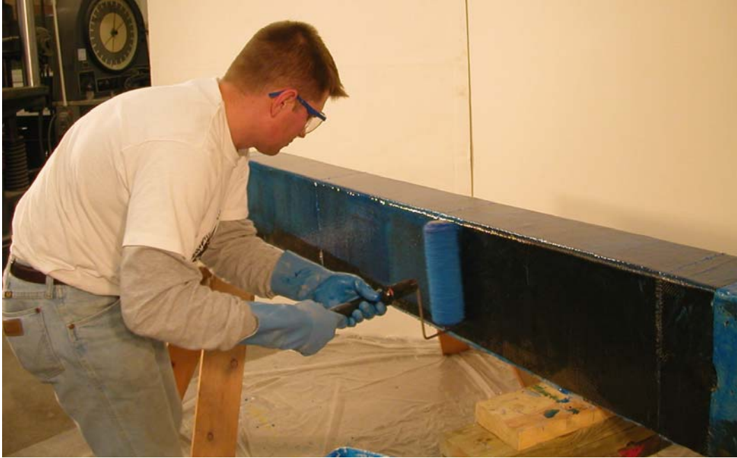
Figure A.51 – A final layer of saturant was applied to the beams on top of the shear reinforcement fabric. The saturant was applied generously to ensure the fabric was fully saturated.
