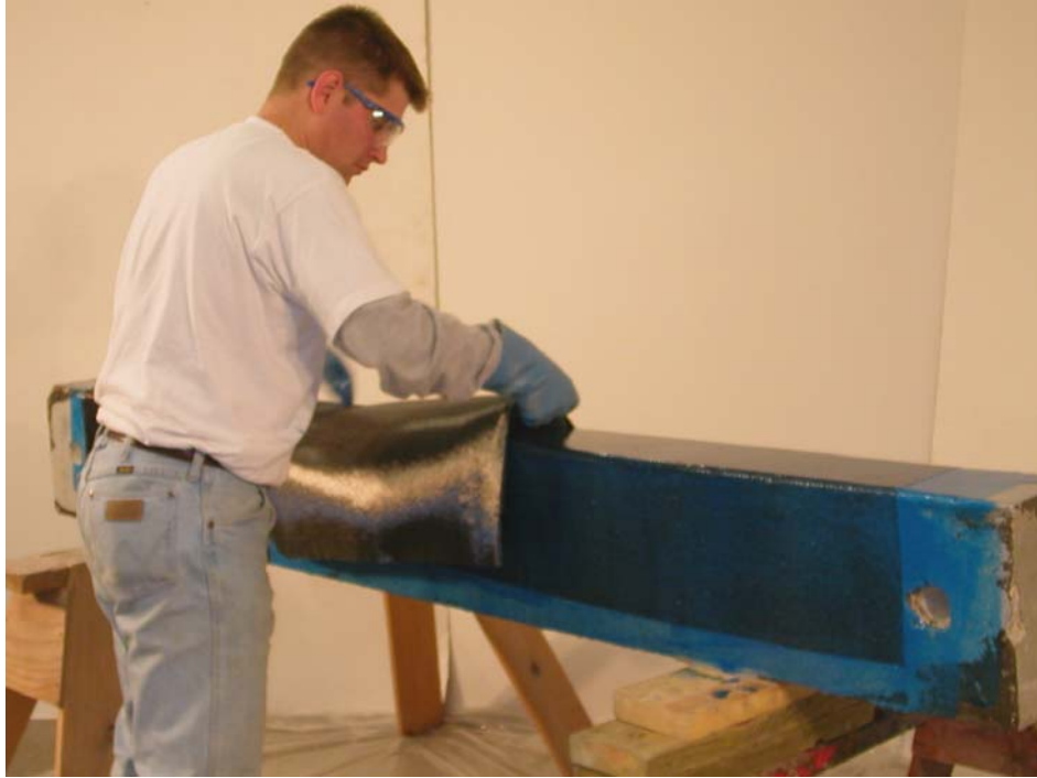
Figure A.49 – The second layer of carbon fiber fabric was applied on top of the fully saturated longitudinally oriented fabric. The second layer of fabric ran perpendicular to the beam's primary axis to provide shear reinforcement.
