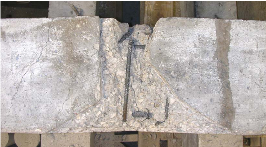
Figure A.29 – The area within the cut edges was scrubbed using a wire brush and pressurized air to ensure it was free of any loose material prior to placing the repair mortar.
