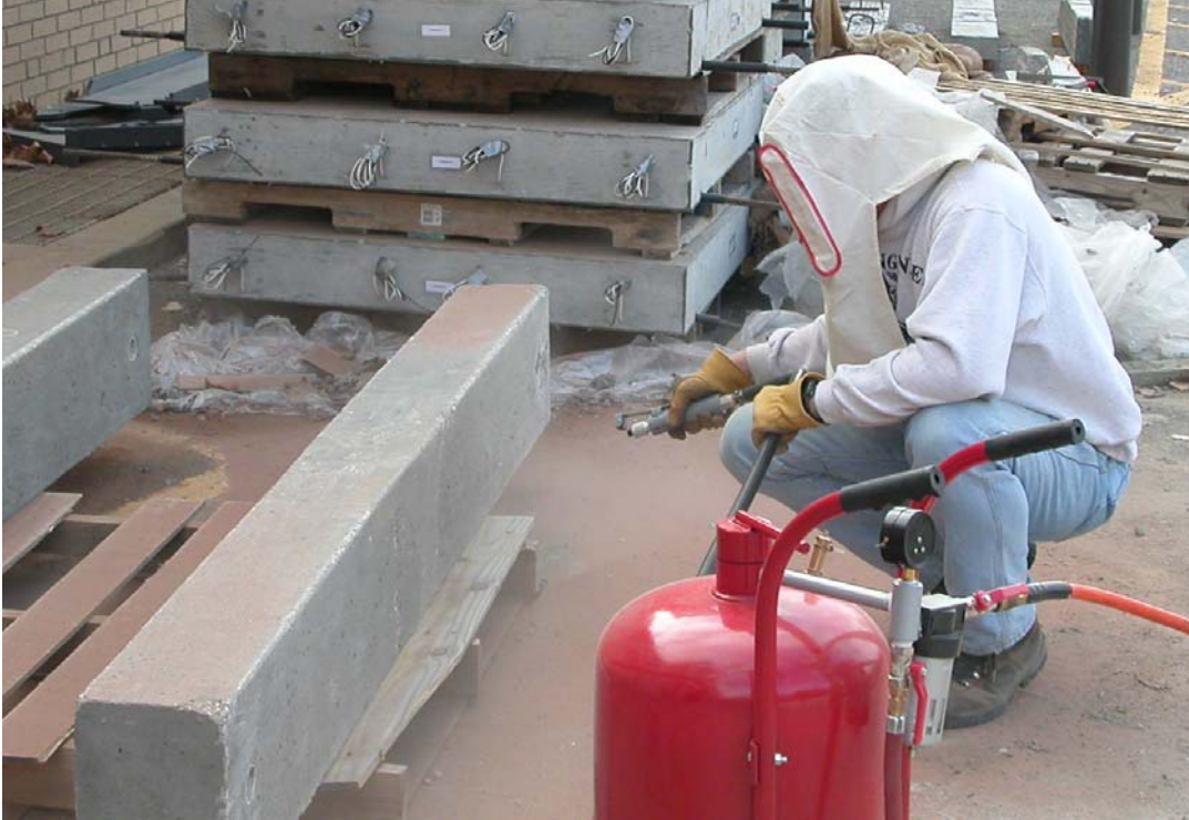
Figure A.34 – Beams 2A and 4A were sandblasted prior to application of the FRP Primer to remove any surface contaminants and prepare the surface for the epoxy primer. Safety precautions, to include no exposed skin and wearing of a hood, must be taken when sandblasting.
