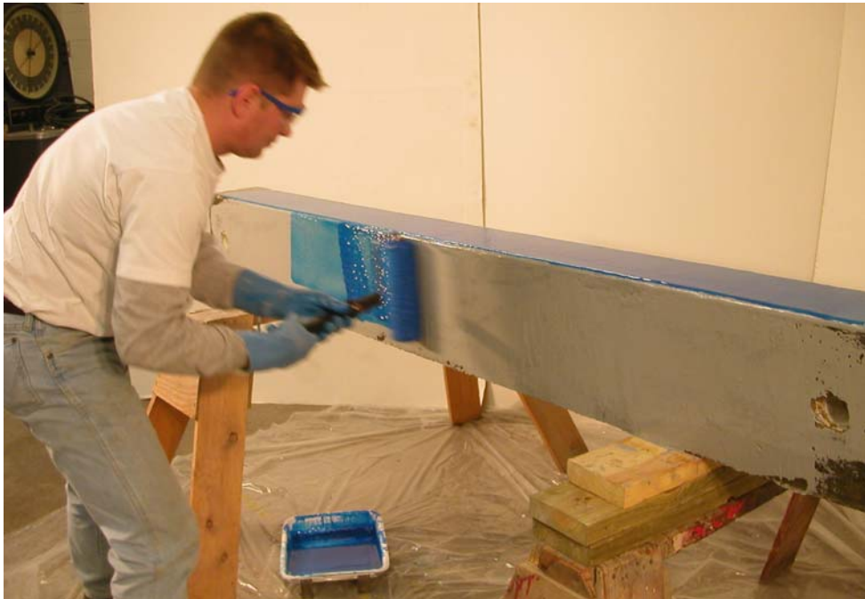
Figure A.46 –The MBrace Saturant was applied to each beam using a medium nap roller.
