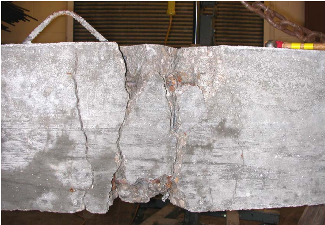
Figure A.24 –This is the outside face of beam 3B after all loose concrete has been removed.
