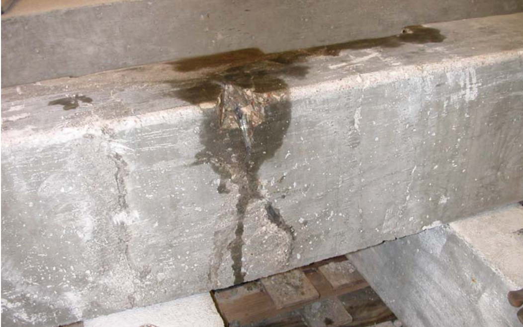
Figure A.32 – The damage at the center of the bottom edge from Figure A- 30 after being cut out.
