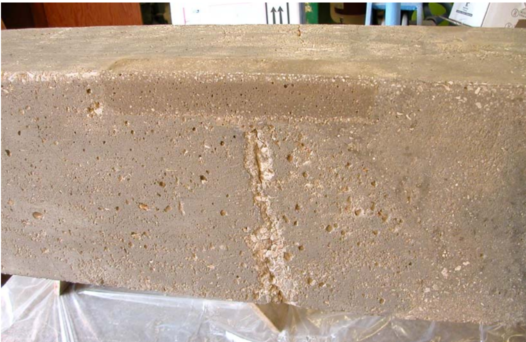
Figure A.33 – The repaired damage of the edge used high-strength repair mortar without any aggregate added. The vertical spalling damage that remains was repaired using the epoxy putty because it was less than \frac{1}{4} in. (6 mm) in depth.
