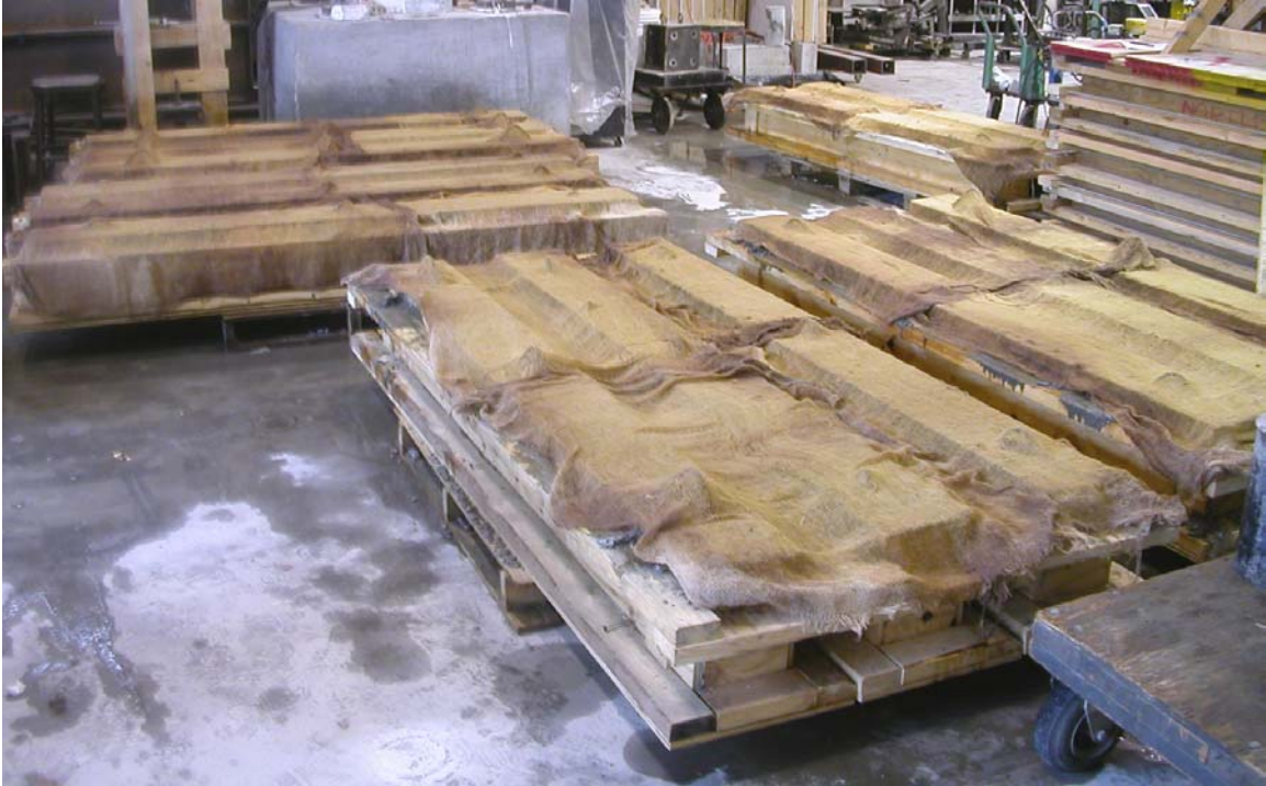
Figure A.5 – Forms were covered with wet burlap following the placement of the concrete to ensure proper curing.
