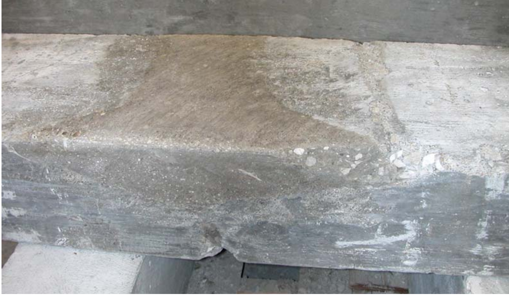
Figure A.30 – Beam 2A after the repair mortar has cured. Because the damaged area was greater than 1 in. (25 mm) in depth, ½ in. (13 mm) max size limestone aggregate was added to the mortar. Note the beam still has remaining damage at the center of the bottom edge and on the right side of the top front edge.
