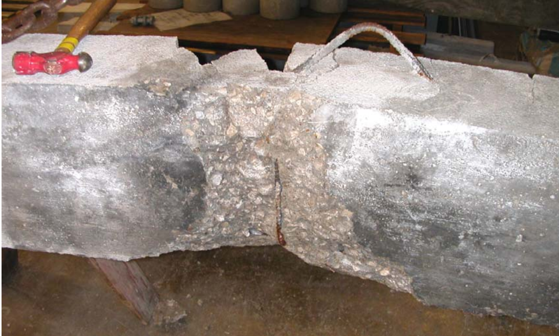
Figure A.23 – The beams were all brought back to the lab where the crushed concrete was removed using a hammer and chisel. This is the inside face of beam 3B after all crushed concrete has been removed.
