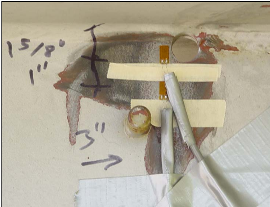
Figure C-2 Installed Gage (Prior to Environmental Protection)
