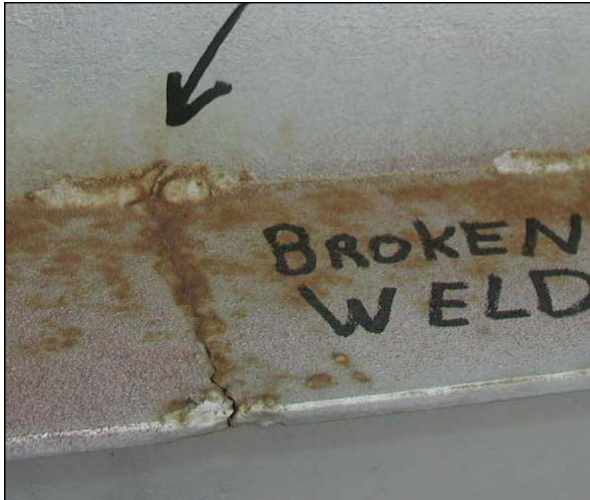
Figure 2-17 Longitudinal Stiffener Crack
