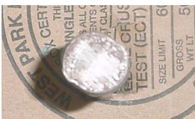
Figure 3.42 – SMI-nc anode bar after removal of mortar, at 15 weeks, showing corrosion products that formed at the unprotected end.
