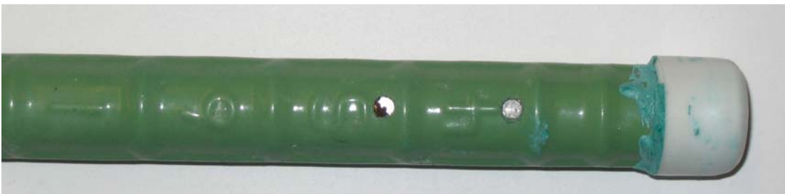
Figure 3.69 – Bare ECR(Valspar) anode bar, at 15 weeks, showing corrosion products that formed at drilled holes.
