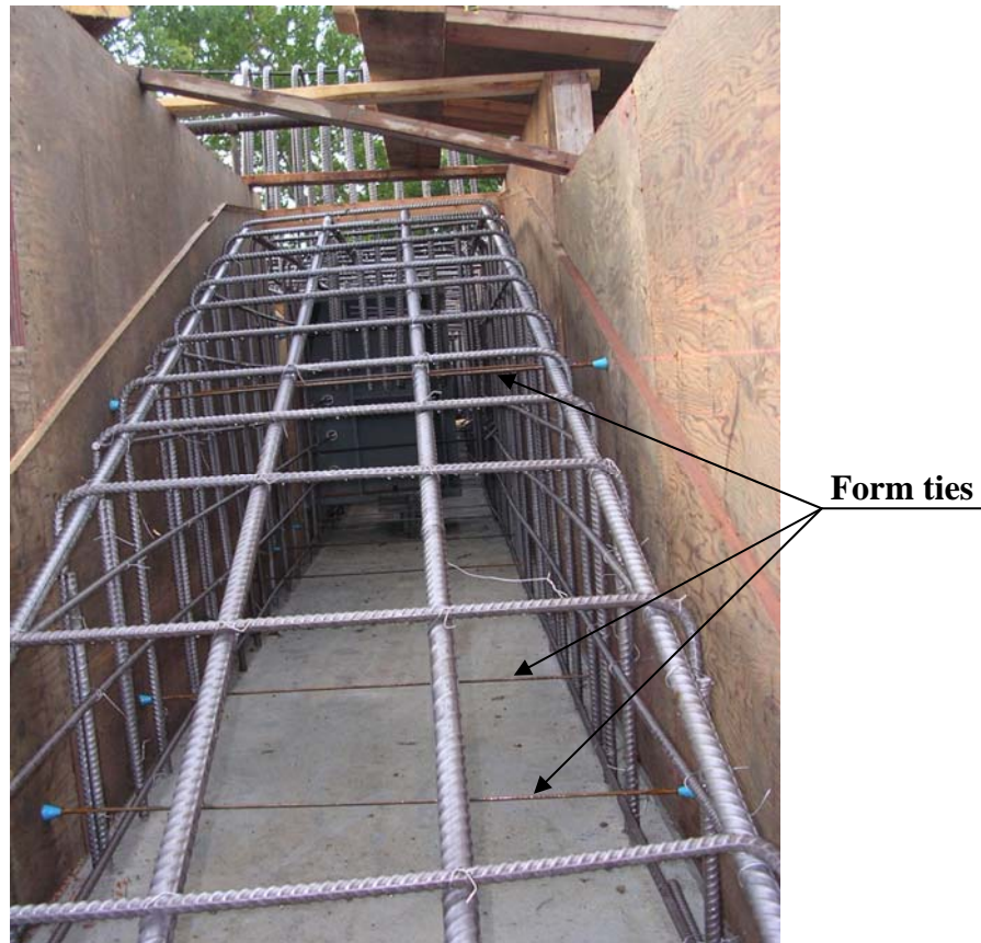
Figure 3.201 – Reinforcing bar cage at the east abutment for the Mission Creek Bridge
