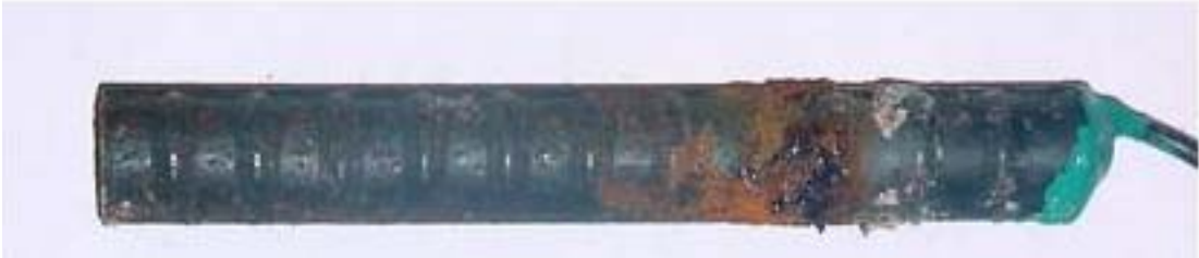
Figure 3.7 – Bare bar specimen. Conventional steel anode bar showing corrosion products that formed at the surface of the solution at week 15.
