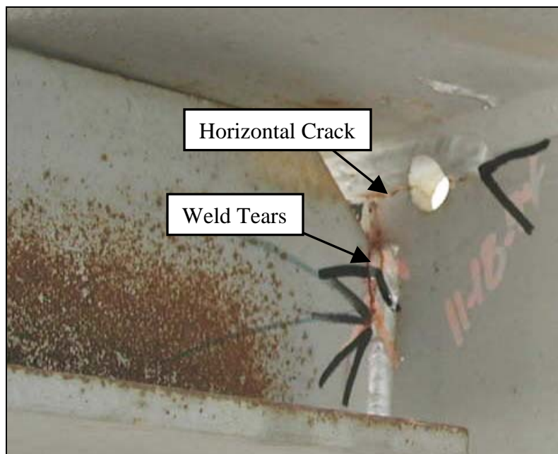
Figure 2-4: Web-Gap Cracking Patterns (Picture)
