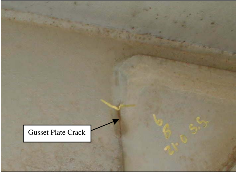
Figure 2-7: Gusset Plate Cracking Patterns (Picture)
