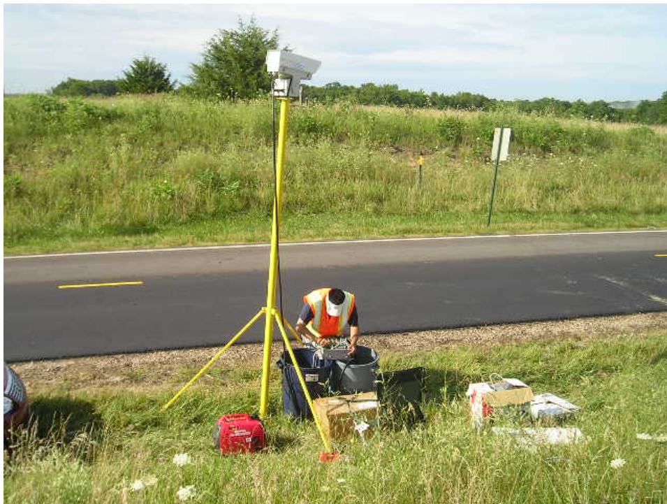
Fig. 18. Connecting the data processor with the camera and AC transformer
