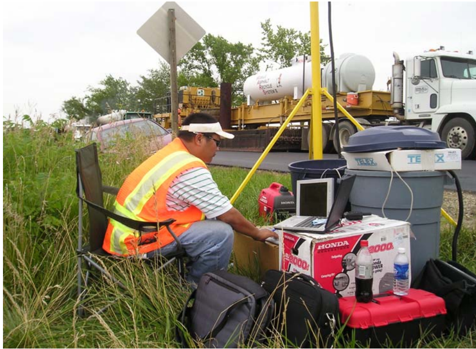
Fig. 19. Operating the system
