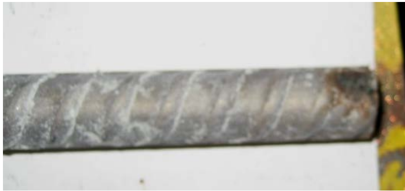
Figure 94c: Top bar from cracked beam specimen 2 containing 2304 stainless steel after autopsy, showing corrosion product near the end of the top bar (close up)
