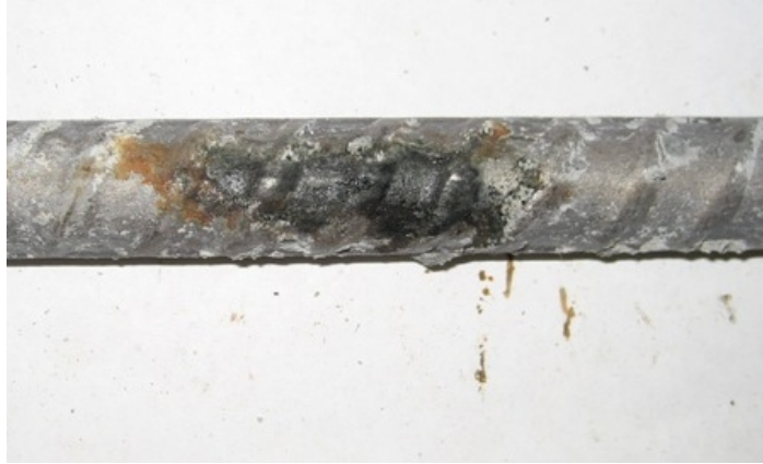
Figure 94b: Top bar from cracked beam specimen 1 containing 2304 stainless steel after autopsy, showing corrosion product on top bar (close up)
