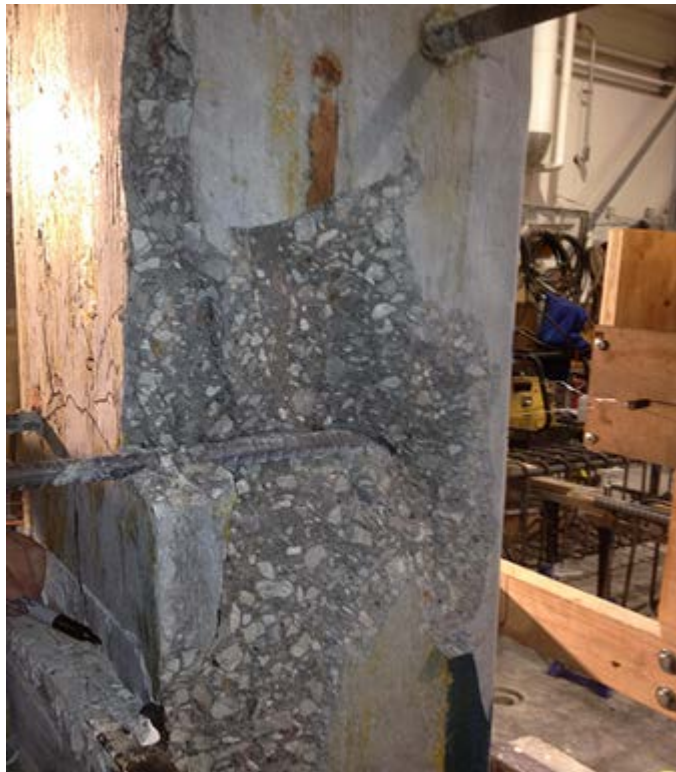
Figure 11 Side blowout failure
