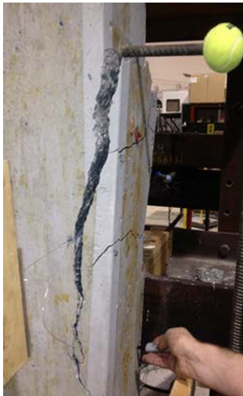
Figure 10 Side splitting failure
