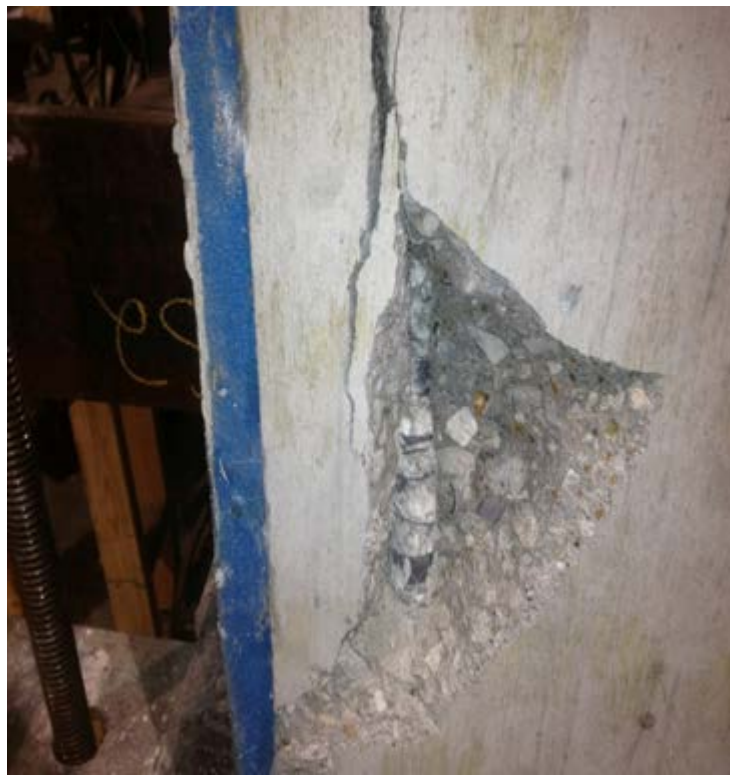
Figure 12 Tail kickout failure
