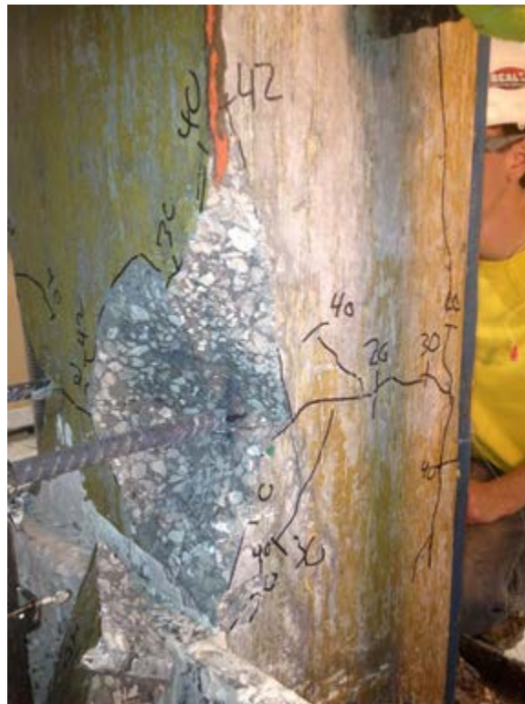
Figure 9 Front blowout failure
