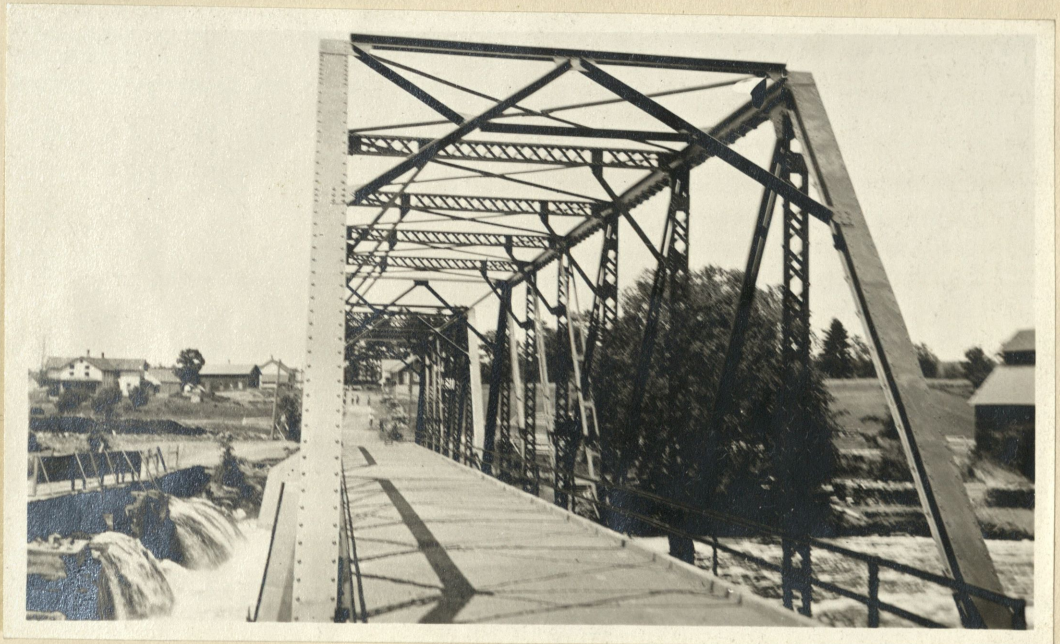
Pella Village Bridge, Shawano County. Two spans of 112 feet 16 feet roadway. Cost $8172.
