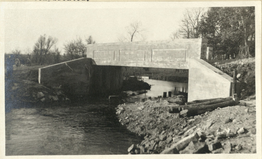
Funkelein Bridge, Town of Christiana, Dane County. Through concrete girders, span 36 feet, roadway 18 feet, skewed 30 degrees. Cost $2340. This is a very easy type of structure to build on a skew. Note the crooked channel of the stream.
