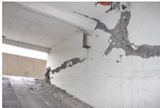
Figure 18. Wall panel with inclined cracks under stack of openings and between anchorage zones of boundary reinforcement from upper stories, Centro Mayor Building, Concepción. Photo credit: J. Moehle, http://nees.org/resources/3111 .)
