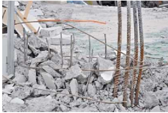
Figure 11. Wall at axes A and 8 (base of the first story), 16 March 2010. Photo credit: G. Alarcón.
