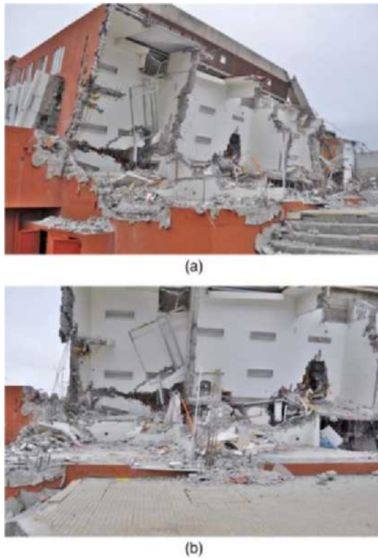
Figure 5. Damage photos for the first story: (a) damage in the first story (view from northwest); (b) observed shift of walls toward the south (view from west). Photo credit: E. Fierro and A. Iruretagoyena.
