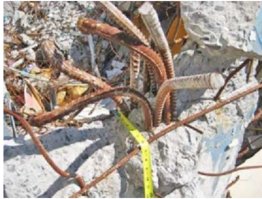
Figure 23. Surviving lap splices.
