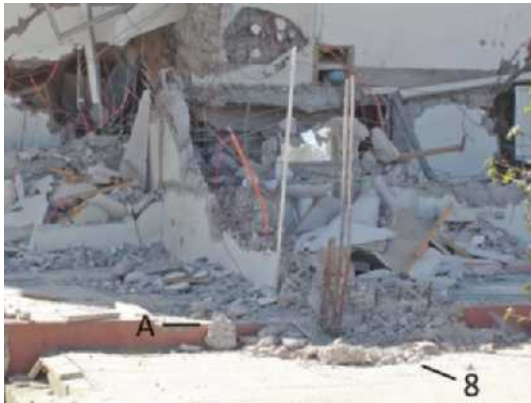
Figure 10. Wall along axis 8 (two of the vertical bars in the foreground had been cut for testing), 29 March 2010.
