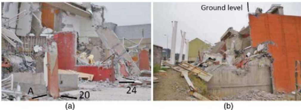
Figure 13. Damage photos before intervention: (a) Axis 24 (view from northwest); (b) axis 35 (view from south). Photo credit: IDIEM.
