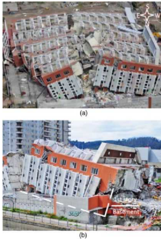
Figure 4. General photos for the Alto Río Building: (a) the Alto Río building after collapse (from http://skyscraperpage.com/cities/?buildingID=85186 ); (b) the damage view from north.
