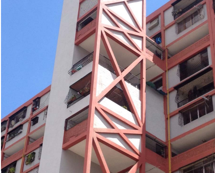
Figure V-9 Residents have built over the roof connecting the elevator tower with the building
