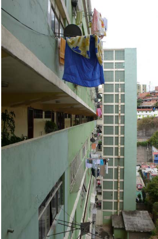
Figure V-8. Cerro Grande back facade. The concentration of props has created a new layer beyond the limits of the original setup. A broken trash chute is visible in this photo.
