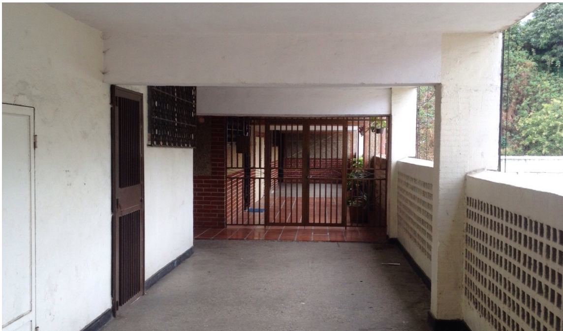
Figure V-12 A group of residents closed a section of the hallway by installing bars and gates. The residents also changed the flooring to personalize and territorialize the corridor.
