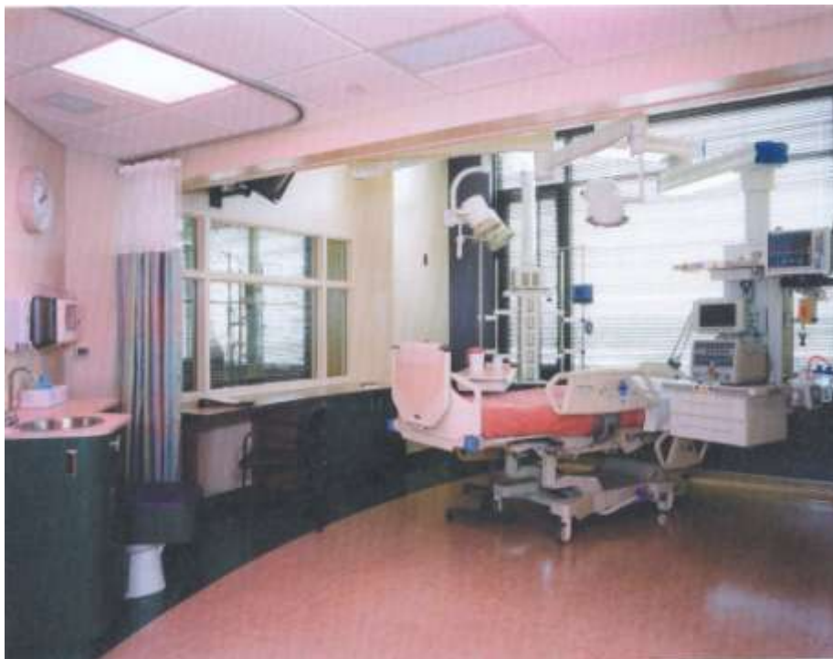
Figure 9: Ceiling-mounted boom in a patient room.
