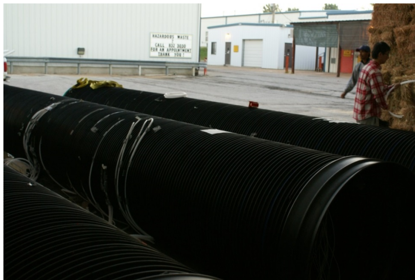
FIGURE 5.1 Test SRHDPE pipes with bell and spigot joints in the field test
