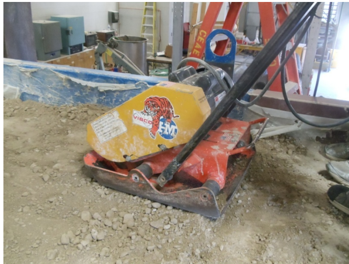
FIGURE 4.20 Compaction of base course using the vibratory plate compactor in Test Section 1
