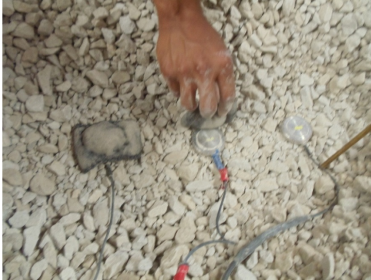
FIGURE 4.23 Earth pressure cells at the crown in Test Section 3
