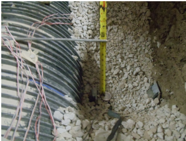
FIGURE 4.22 Earth pressure cells at the springline in Test Section 3
