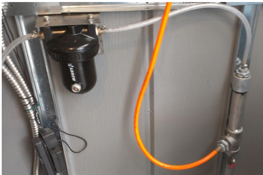
Figure 5 - Air dryer (left) and custom flow separator (right) in line before air controller
