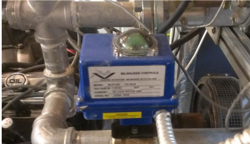
Figure 31 - Backpressure valve with open position indicated
