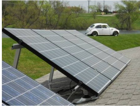
Figure 6: Solar array on the roof of the EcoHawks' design laboratory.
