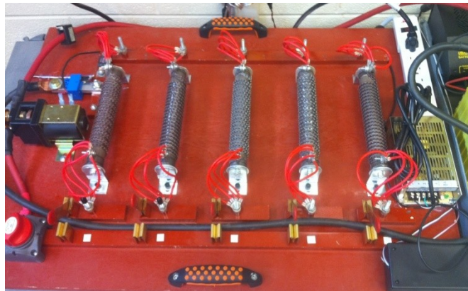
Figure 2: Variable resistive load bank constructed to discharge batteries under adjustable currents.
