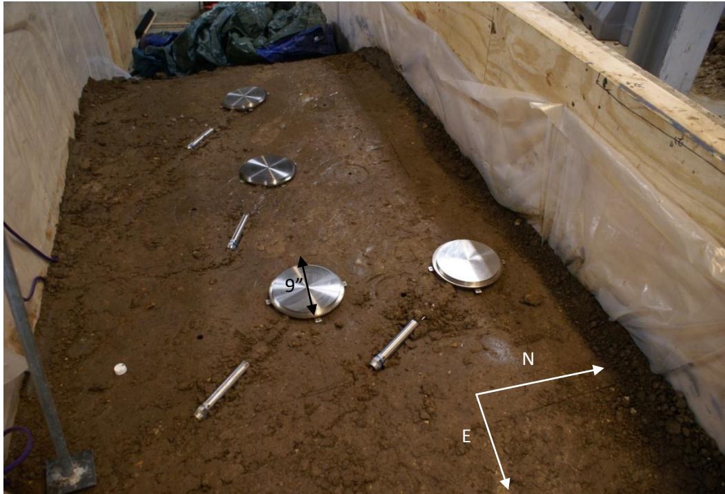
Figure 3.15 Model 3515 circular earth pressure cells during placement
