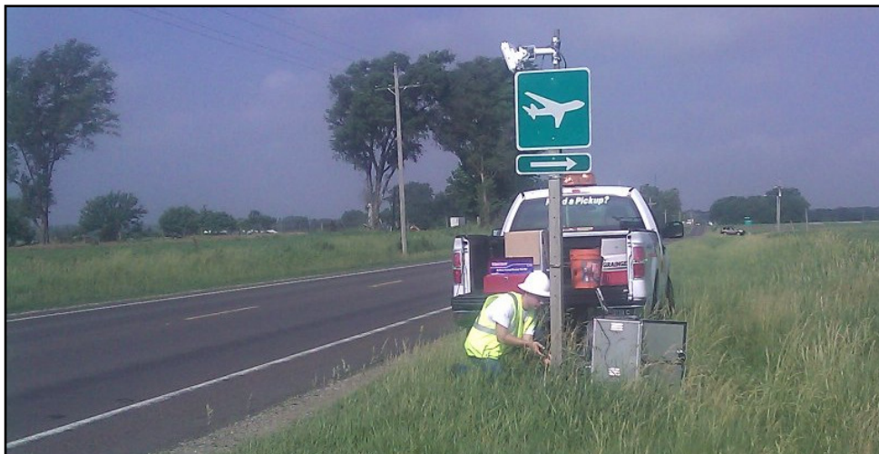
Figure 29 Smartsensor Installed on Signpost with the Cabinet at the Base of the Post
