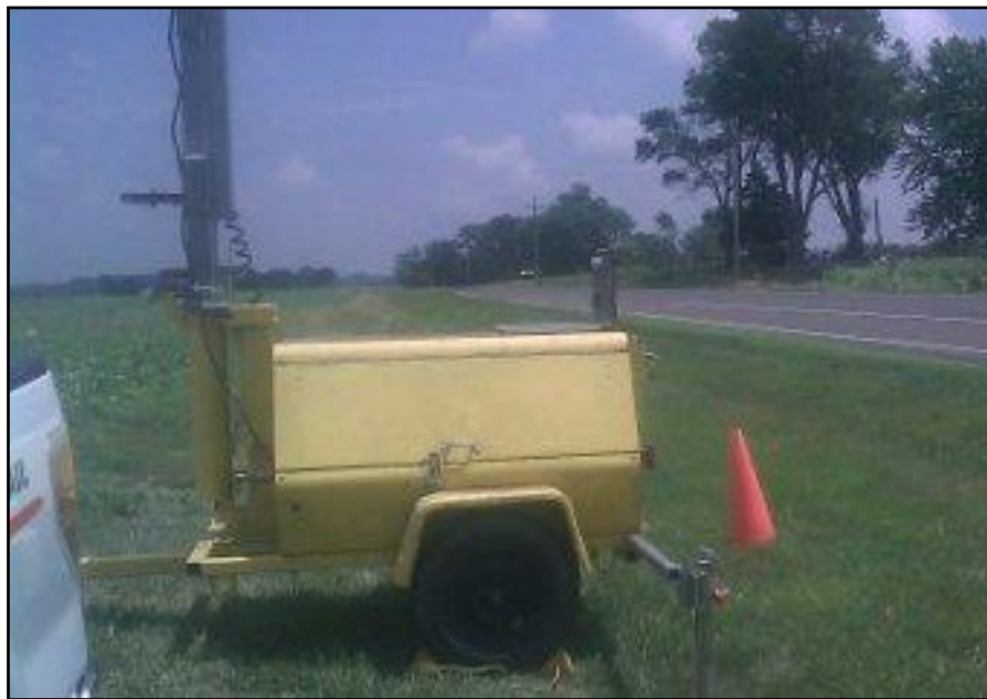
Figure 31 Trailer with Cabinet for the Autoscope System
