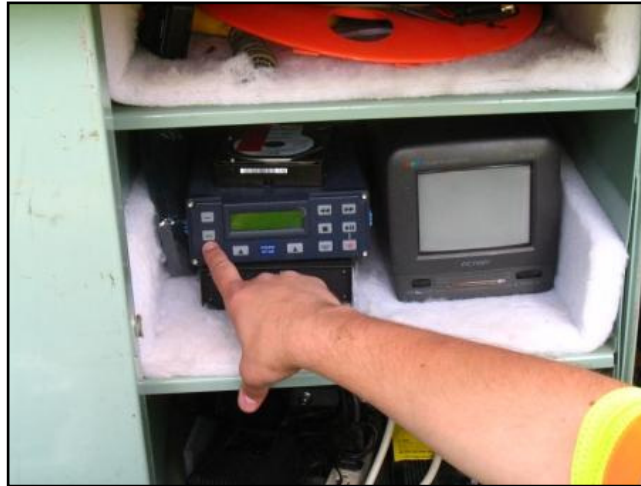
Figure 30 Battery, Recorder, Hard Disk and TV Setup for the Autoscope System
