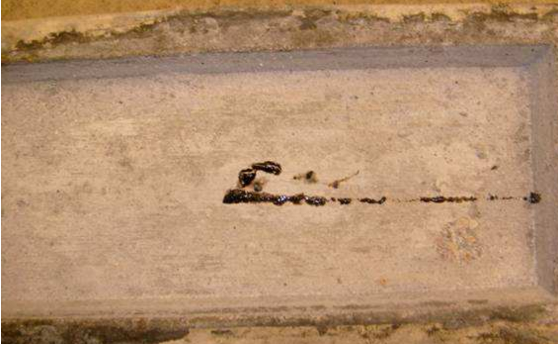
Figure 4.19: Galvanized reinforcement, 25 mm (1 in.) cover. Staining on surface at crack initiation.
