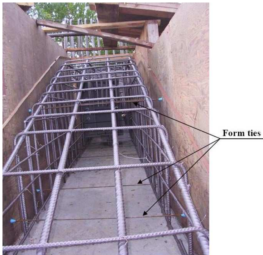
Figure 3.149: Conventional steel form ties in Mission Creek Bridge abutment.
