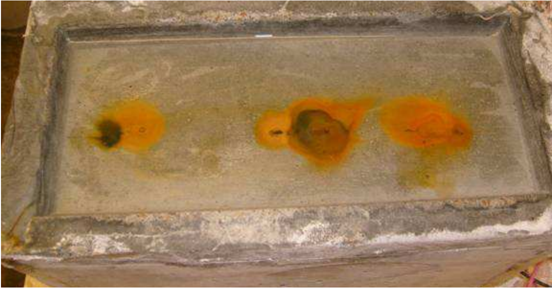
Figure 4.11: Specimen Conv.-1, 25-mm (1-in.) cover. Surface cracking and staining.
