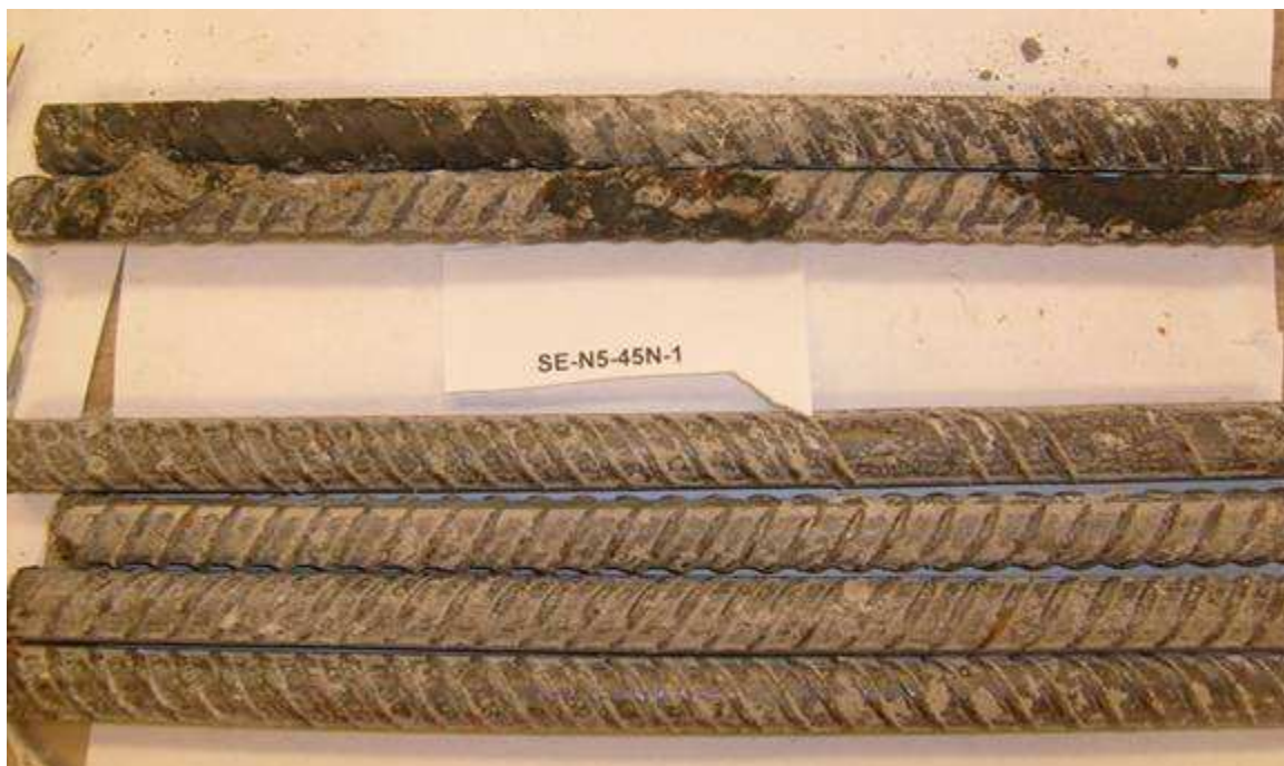
Figure 3.7: Specimen SE-Conv.2-1, 96 weeks. Steel in top mat (above label) and bottom mat (below label).
