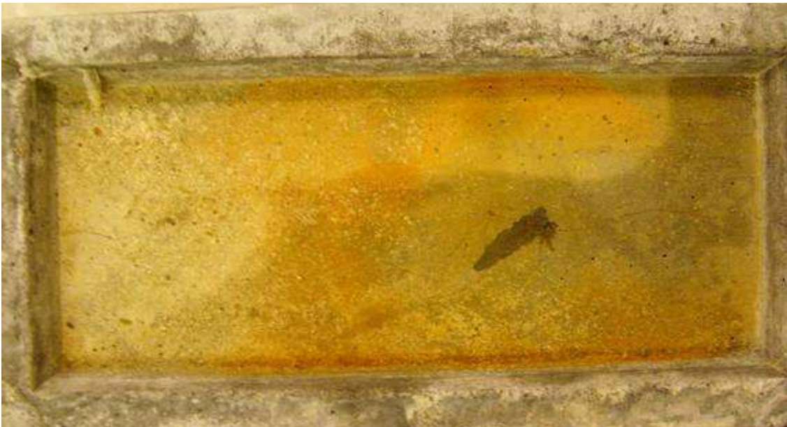
Figure 4.12: Specimen Zn-4, 25-mm (1-in.) cover. Surface cracking and staining.
