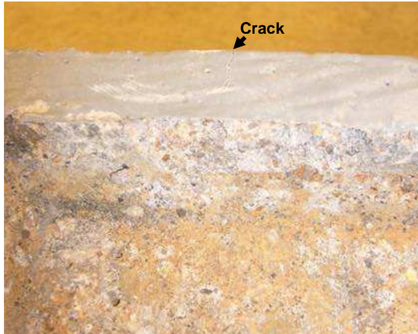
Figure 3.15a: Specimen CB-Conv.2-2 (top surface detail), 96 weeks, showing cracking of the concrete.
