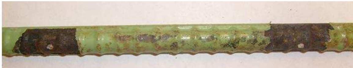
Figure 3.85: FTS-ECR(RH)-C-1, showing total disbondment on a bar from the top mat of steel.
