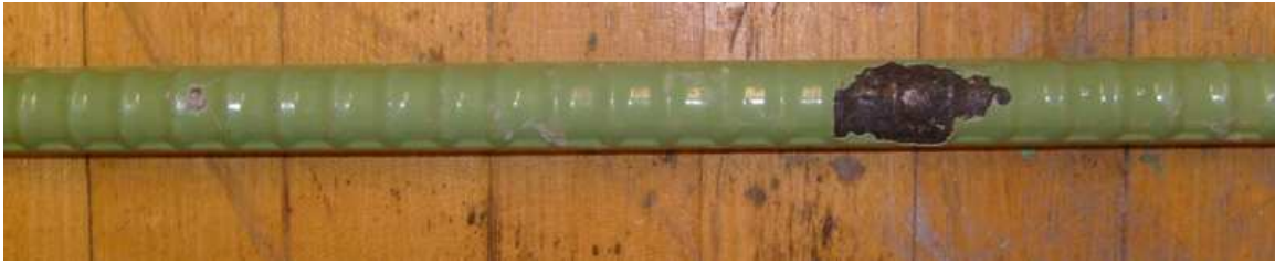
Figure 3.84: FTS-ECR-C-2, showing moderate disbondment on a bar from the top mat of steel.
