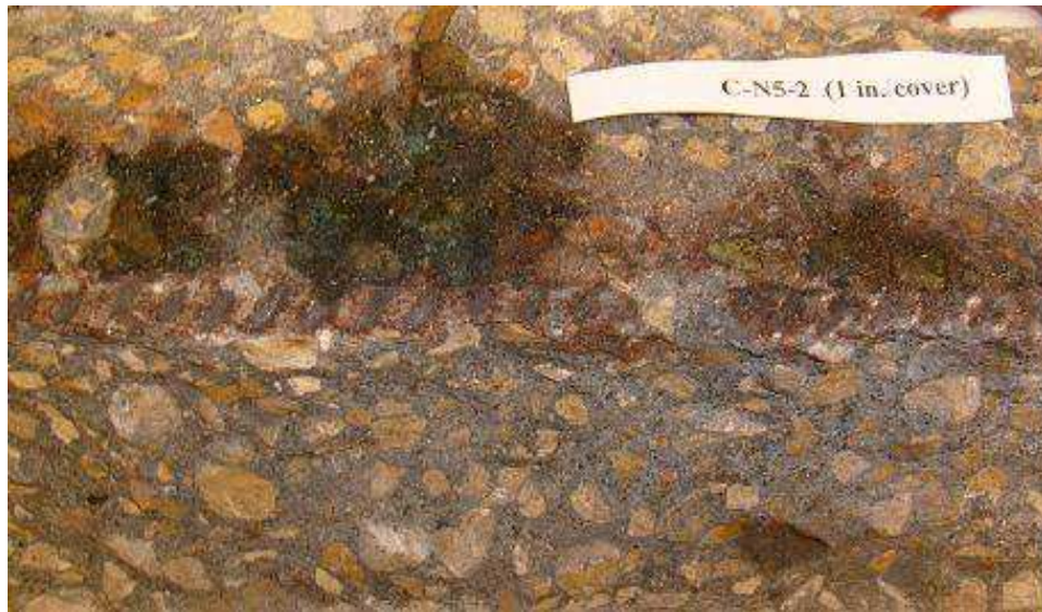
Figure 4.15: Specimen Conv.-2, 25-mm (1-in.) cover. Top view; concrete at the depth of reinforcement. Photos taken immediately after autopsy.
