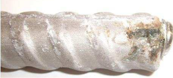
Figure 3.123: CB-DCB(2205p)-2, 240 weeks. Corrosion near bar end.
