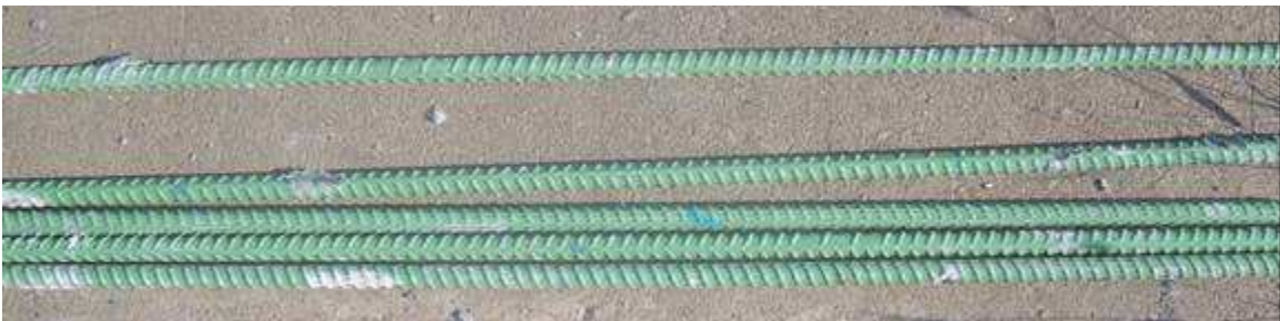
Figure 3.146: Specimen FTS-DCB(ECR)-1, selected bars from top mat of steel showing no corrosion. (White marks are jackhammer damage)
