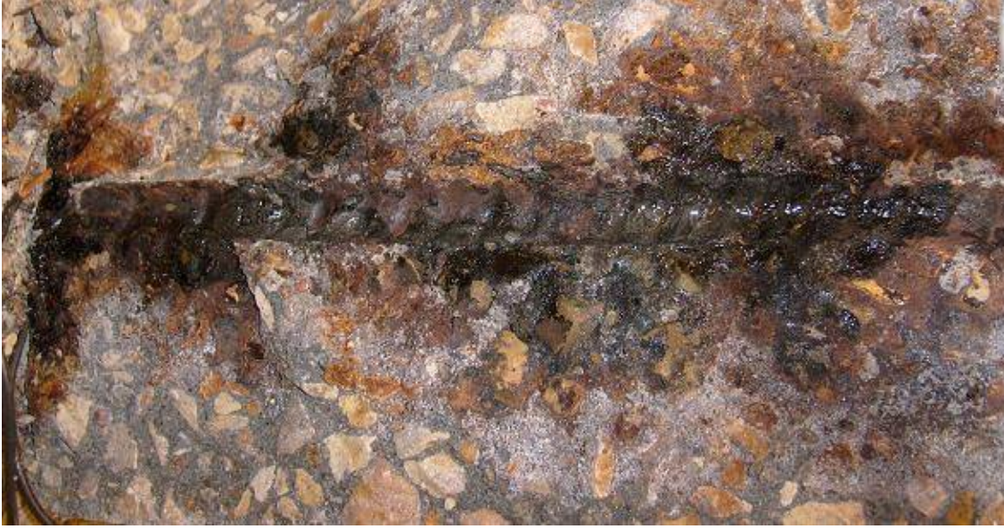
Figure 4.18: Specimen Zn-4, 25 mm (1 in.) cover. Top view; specimen split at depth of reinforcement. Photos taken immediately after autopsy.
