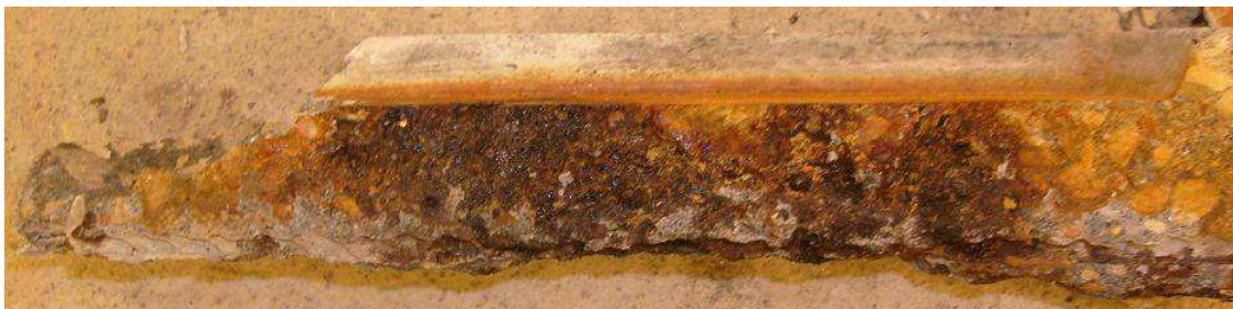
Figure 4.17: Specimen Zn-4, 25 mm (1 in.) cover. Side view; plane of crack visible above reinforcement. Photos taken immediately after autopsy.
