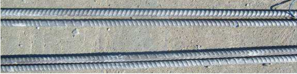
Figure 3.147: Specimen FTS-DCB(2205p)-1, selected bars from top mat of steel showing no corrosion.
